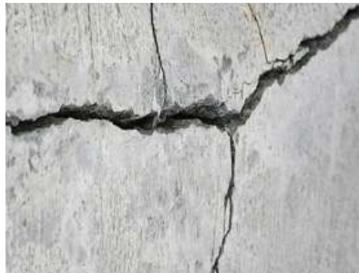
© stone crack Fotolia #36569926
